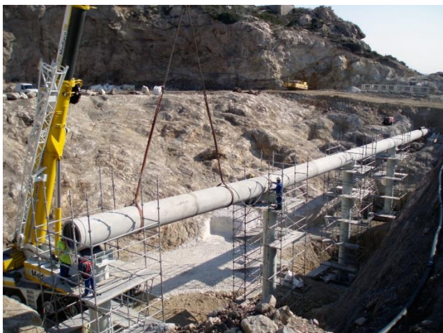
Ø 800: Marseilles (France) Free span of 12,3m
