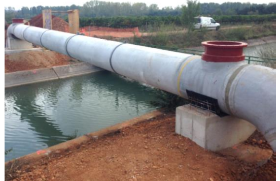
Ø 800mm : CNM Nîmes Costières (France) free span of 15,6 m test pressure: 10bar
